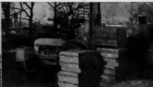
Self-palletized brick pack speeds up deliveries over former manual brick-by-brick loading. Idea 535
